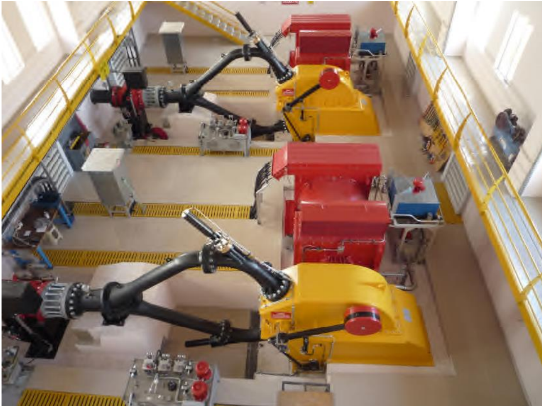
Figure 8 - Horizontal Pelton turbine plant in Turkey (image provided by WKV)
