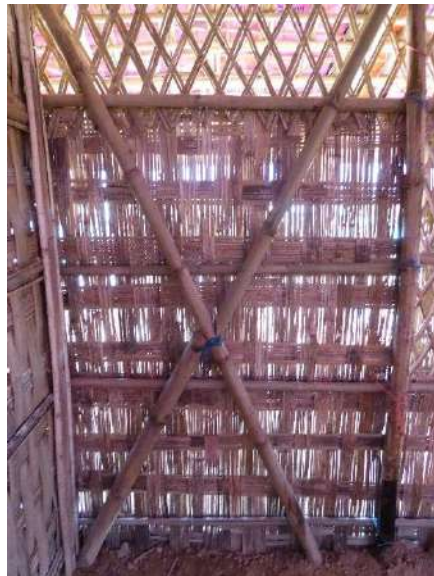
Above: diagonal bracing has very little if any capacity because of weak and loose connections at both ends
