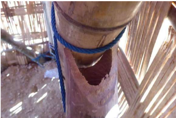
Above: ill-fitting bamboo brace
