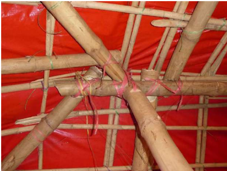
Above: existing connection using plastic packaging strips which is very loose
