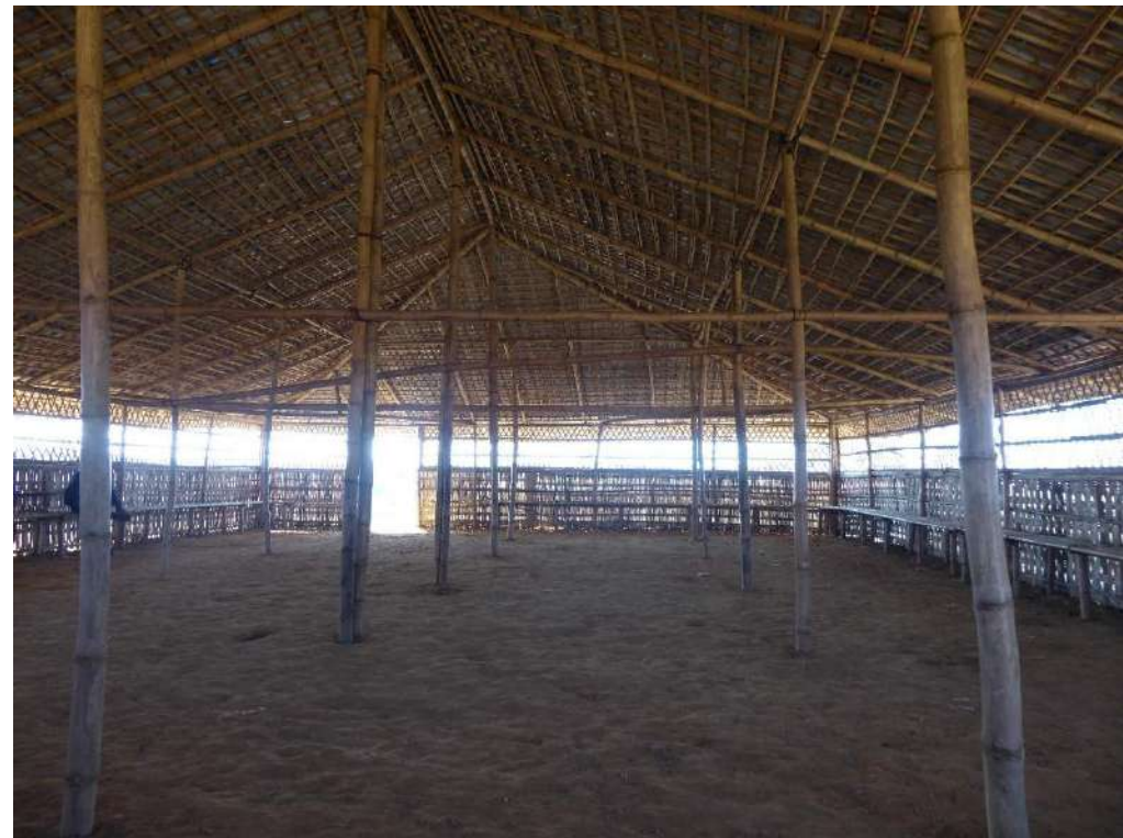
Large mosque with no internal bracing and long roof spans. This is likely to completely fail in even small winds.
