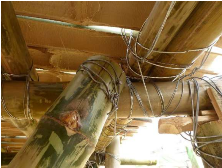
Above: diagonal bracing has very little if any capacity because of weak and loose connections at end
