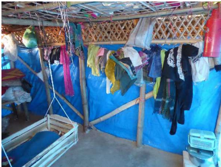
Above: diagonal bracing has very little if any capacity because of the weak and loose connections at each end
