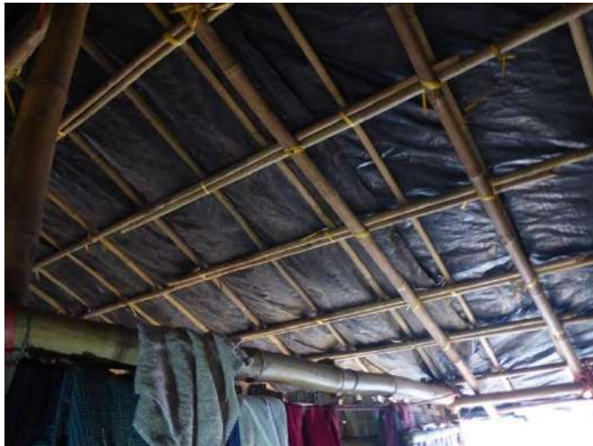
Above: borak as rafter has little benefit, double layer of muli has little benefit
