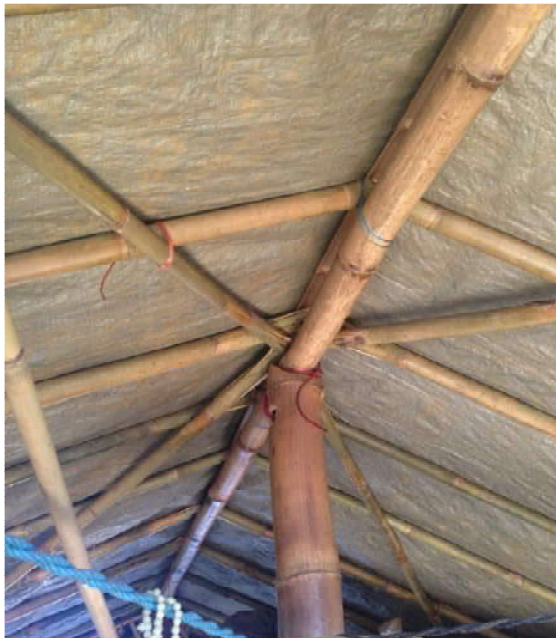
Above: none or ineffective bracing seen in shelters
