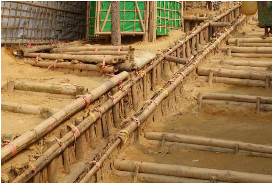
Above: Raised drainage channel limiting water entry and overall capacity in high flow
