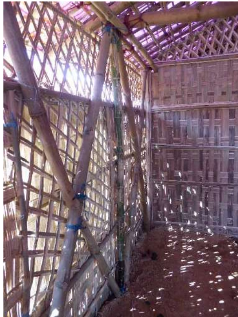
Above: small diameter or split bamboo being used for eaves is weak.
