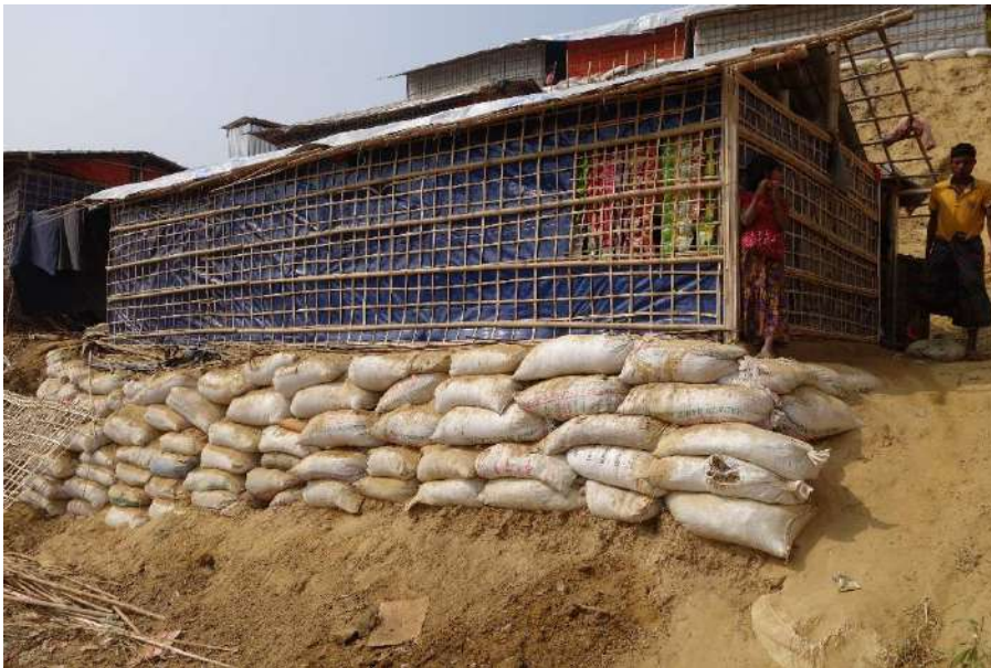
Above: Sand bag retaining wall without adequate anchoring to slope
