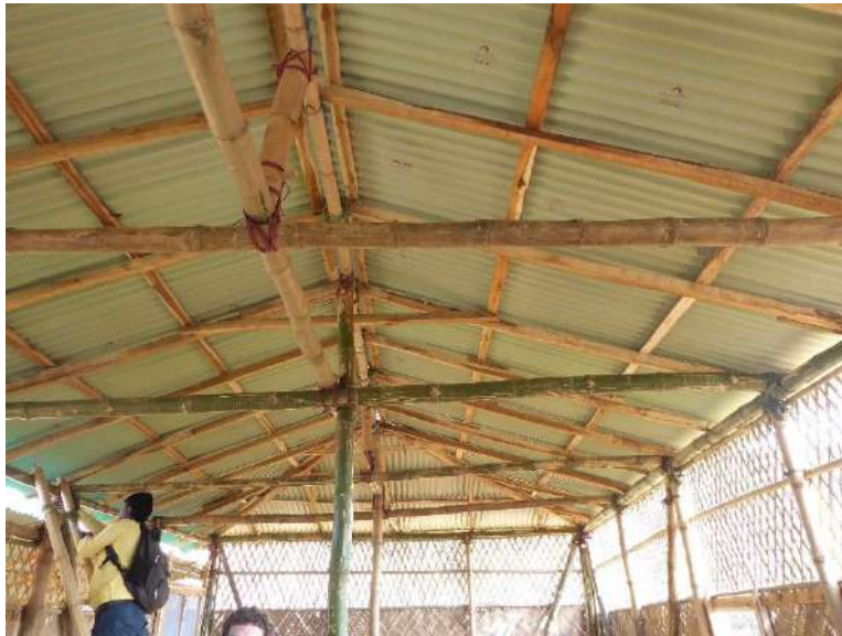
Left: building missing stability in short direction
