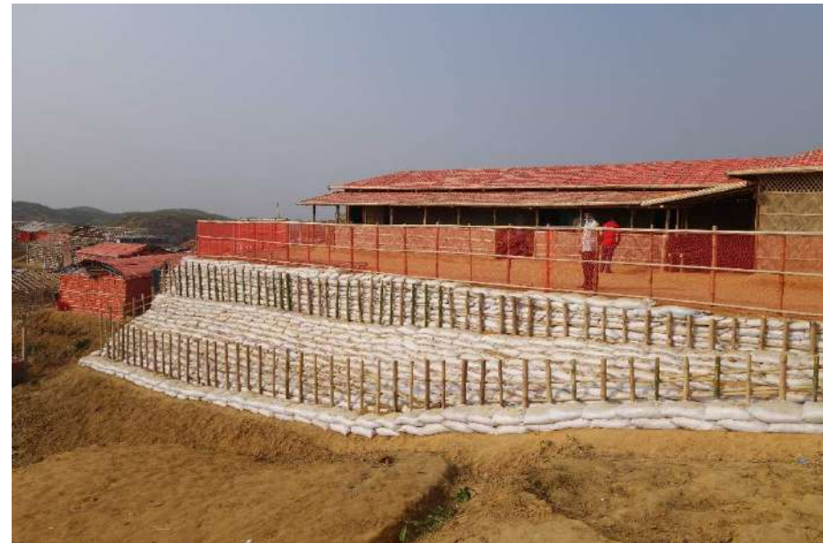
Above: Ensure large walls are tied to slope with footings and/or nails
