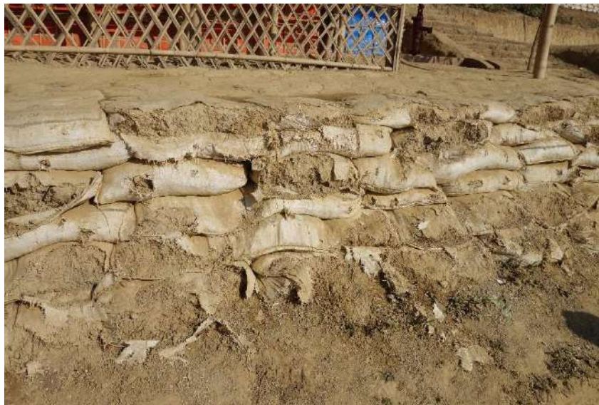
Above: rapid degradation of sand bags and failure of slope
