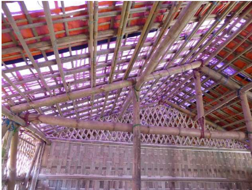
Above: no or ineffective plan bracing seen in shelters
