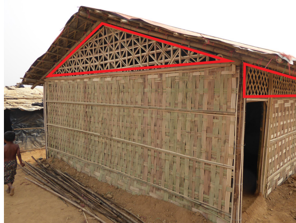
Figure 11: Example of ventilation grids
