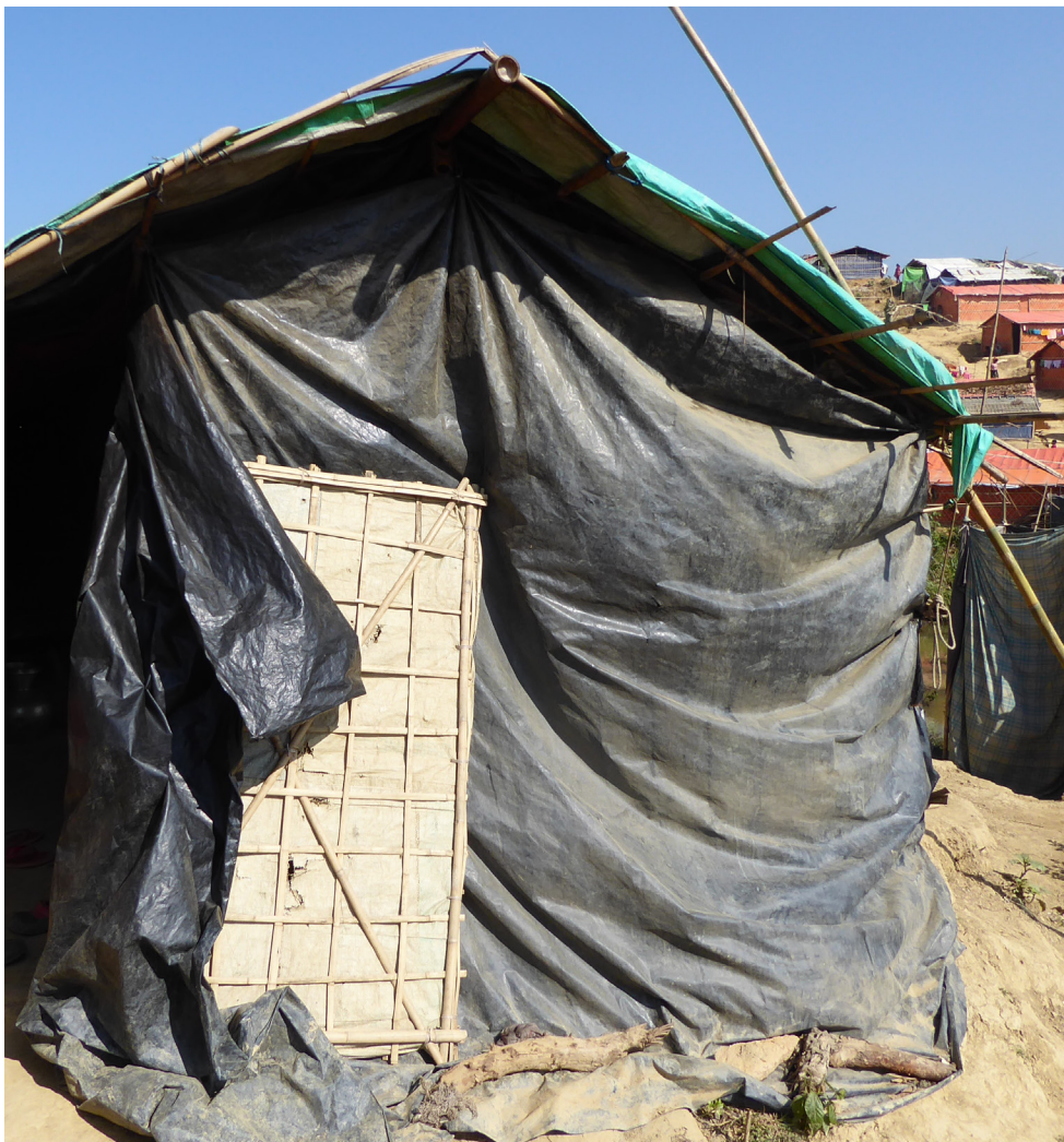
Figure 2: Typical self-built bamboo shelters without technical input - the structural frame is light and not robustly connected, and the plastic sheeting is only loosely connected back to the frame.
