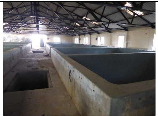
Figure 45: Empty shrimp hatchery in Cox's Bazar could be used for bamboo treatment with boron (Cox's Bazar)
