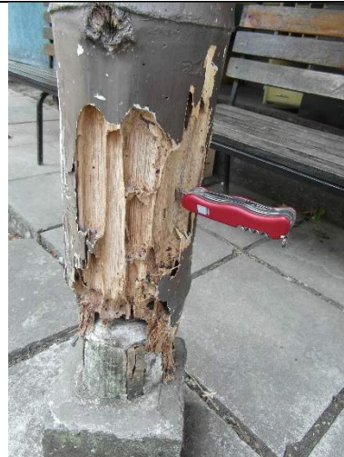
Figure 16: Significant termite damage to bamboo column (Costa Rica)
