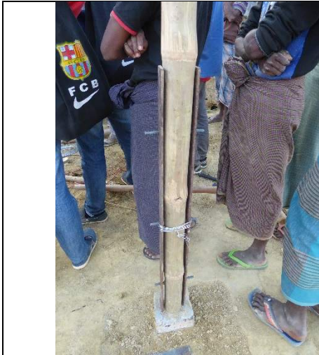
Figure 34: Elevate and separate frame from ground using a concrete footing, with the bamboo sitting on top and bolted to it via a cast in steel plate. Ideally also place a plastic membrane between the concrete and the bamboo (Cox's Bazar)
