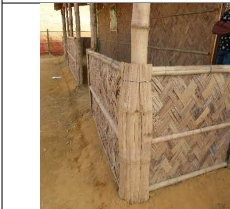
Figure 38: Protect all exposed bamboo from driving rain, such as here using split bamboo to protect a veranda column. Note however this can hide termite tunnels. (Cox's Bazar)
