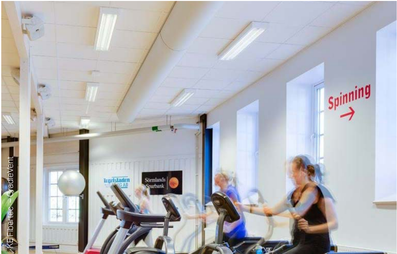
Figure 103: Example of cradle-to-cradle certified textile ductwork, Cradle Vent, used in a health center
