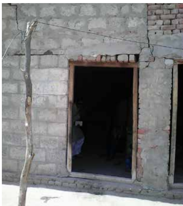
Figure 08: Example of low strength wall
