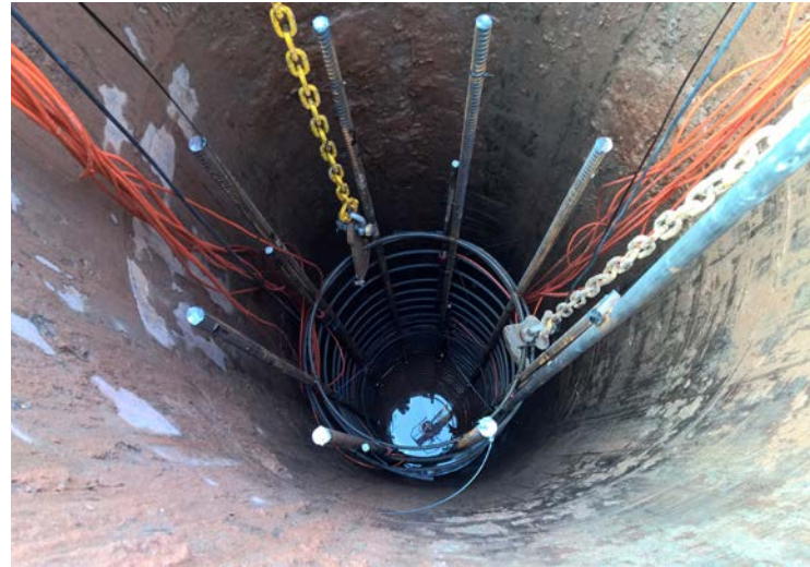
7: The piles were designed to ensure the structure met the settlement criterion, which was more than five times stricter than for a typical building
