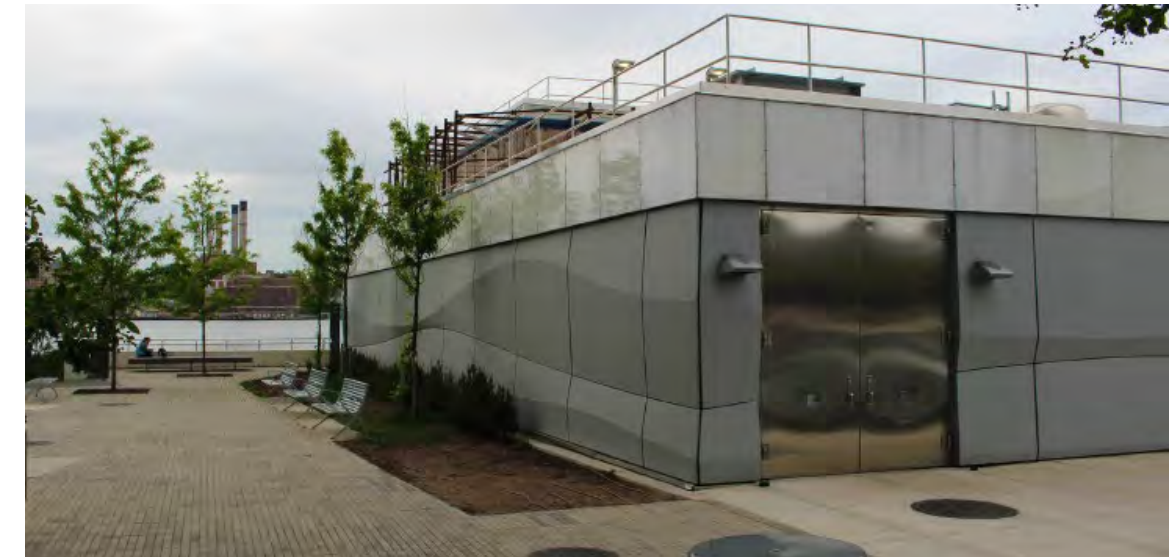
Infrastructure improvements for MTA buildings lying in vulnerable areas included GFRC clad flood walls and a flood resistant door .
