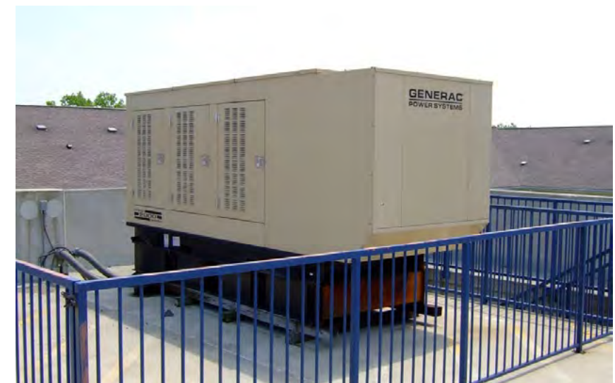
To ensure business continuity, it is essential to safeguard mechanical, electrical, and backup systems. Renovations provide an opportunity to install these systems in locations with a low risk of flooding.
