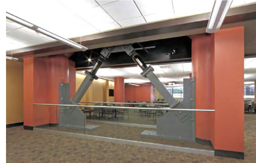
Retrofit of seismic dampers reduces damage from earthquake and provides opportunities to minimize disruption to the office floor plate.
