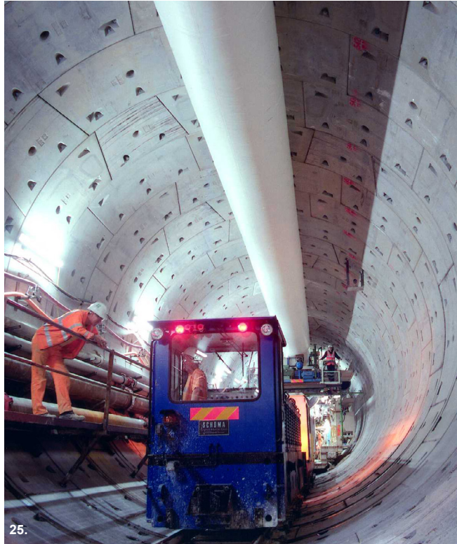
The CTRL tunnel passed under the Thames, necessitating the development of measures to prevent flooding
