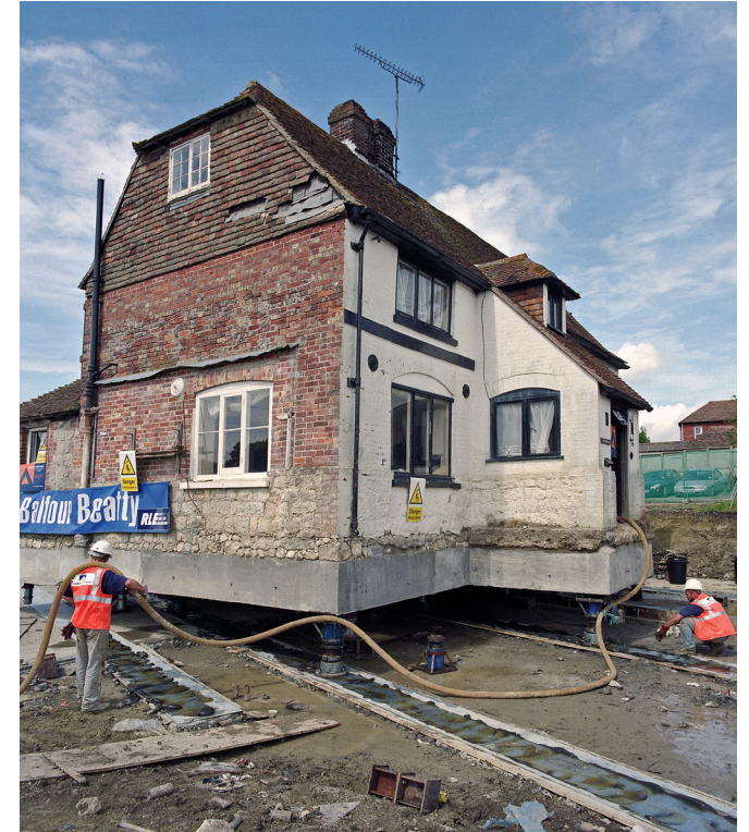
The historic Bridge House in Mersham, which stood on the HS1 route, was slid 80m to a new location
