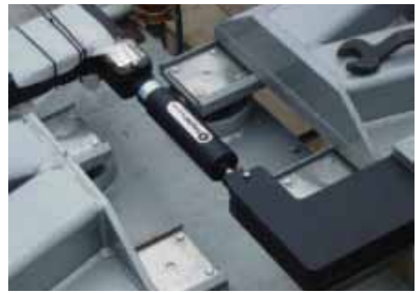
8. Viscous damper under bridge deck.
