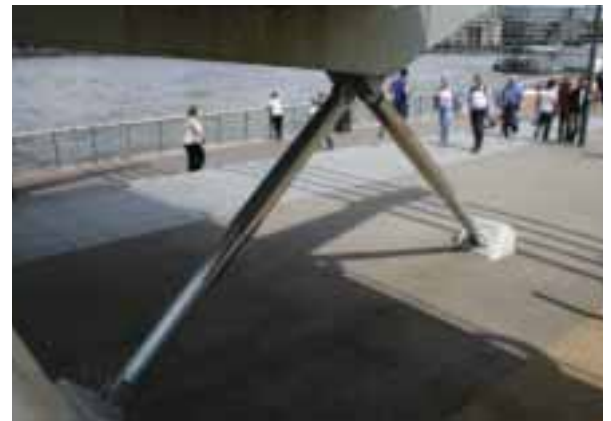
9. Diagonally braced viscous damper under abutment.
