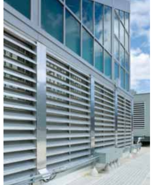
14. Rooftop motorised louvres.
