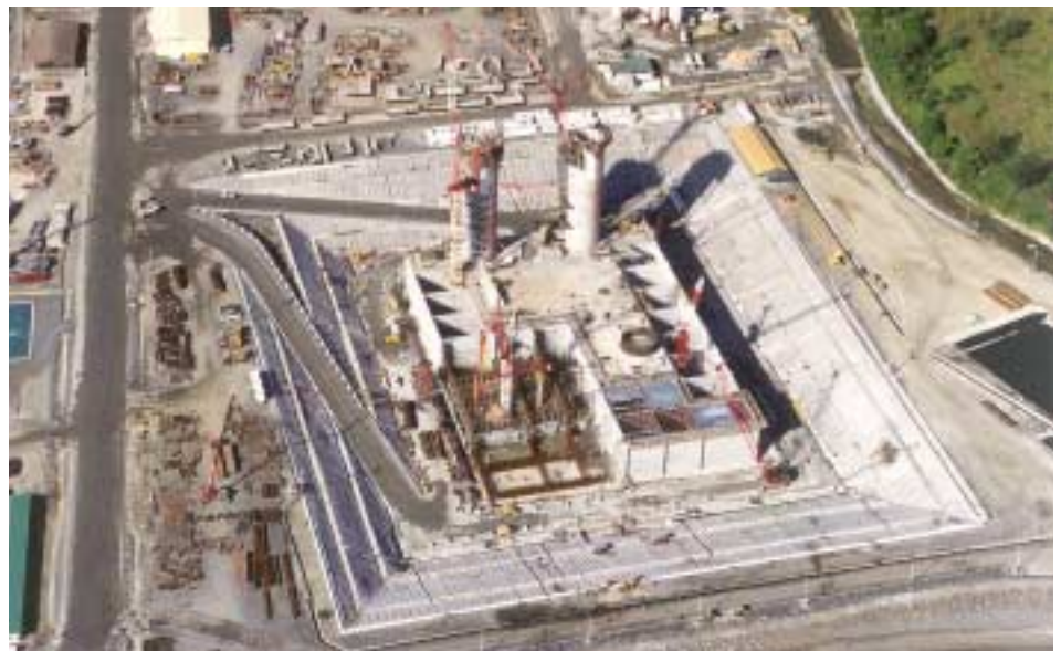
5. The CGS in the casting basin, with slipforming of the base caisson in progress.
