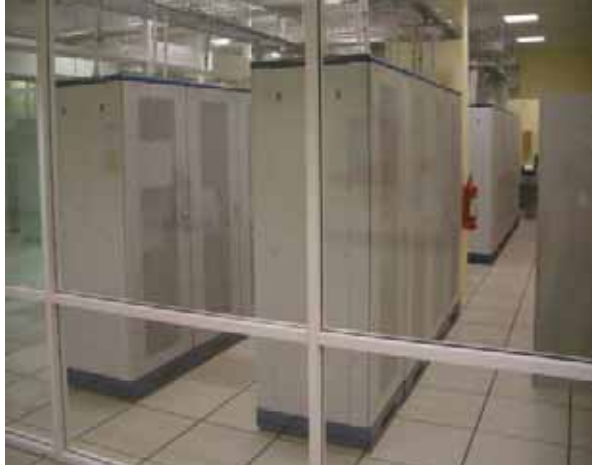
9. The main server room.
