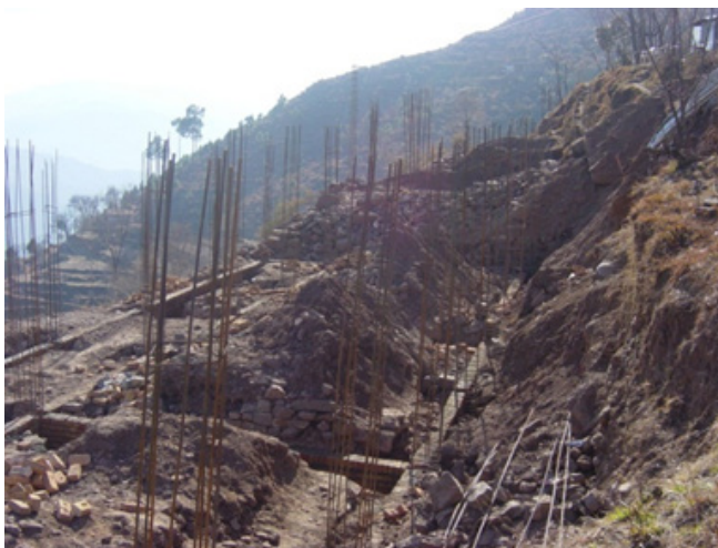
Figure 10b. SCHOOL RECONSTRUCTION, PAKISTAN. Although the school building was designed to reduce vulnerability to earthquakes the risk was still high due to the exposure of the site. Therefore major earthworks were required to protect the school from potential landslides.
