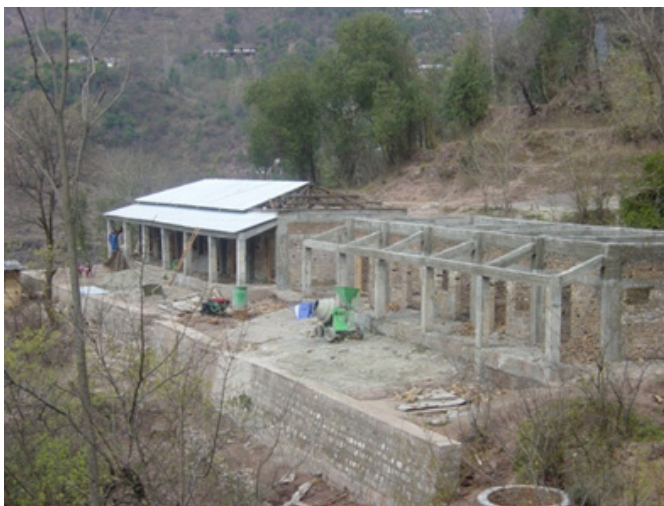
Figure 12a. SCHOOL RECONSTRUCTION IN PAKISTAN. Access to appropriate technical expertise ensured that inadequate seismic detailing was identified and amended during design review.
