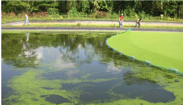
Underperforming wastewater lagoons in Australia
