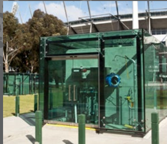
Melbourne Cricket Ground Water Recycling Facility , Victoria, Australia
