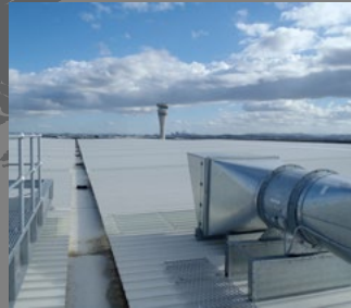
Brisbane Airport Domestic Terminal Recycled Water Supply , Queensland, Australia
