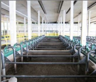
Genting Wastewater Treatment Works, Malaysia
