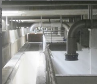
Liwasan Ng Kagitingan at Kaliksan Wastewater Treatment Plant, Manila, the Philippines
