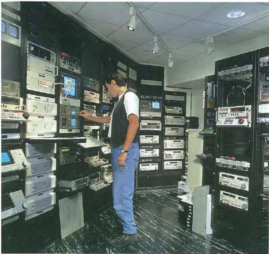
18. Video post-production facility: the Telecine Equipment Room
