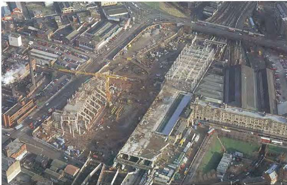
3. Aerial view from west on completion of station work: the Arena is on the left, the listed station entrance façade to the right, and the roof to the 'city room' top right.
