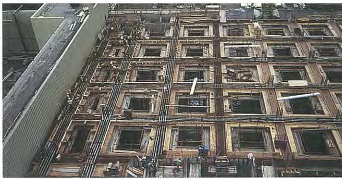
5. Second process building showing the post-tensioned beams and the beam-and-column structure in the open or reserve section.
