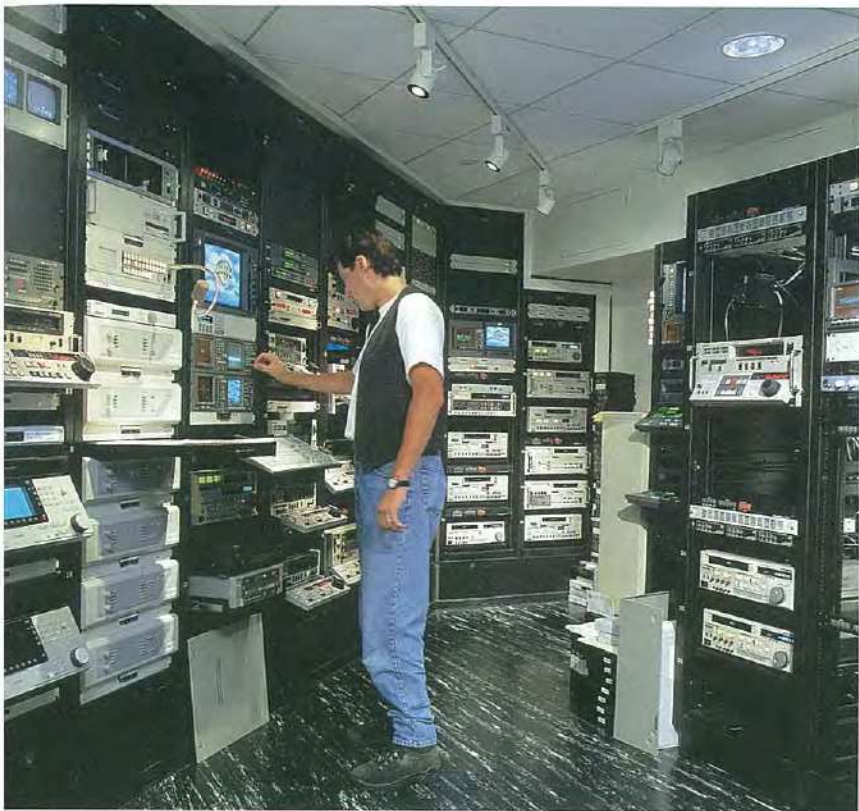
18. Video post-production facility: the Telecine Equipment Room
