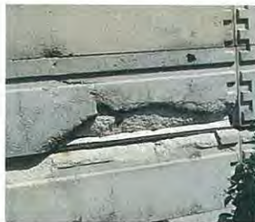
7. Blocks are stack-bonded without mortared joints. Reinforcement is horizontal and vertical in edge grooves, grouted with a fluid cement mortar. Rusting has led to spalling.
