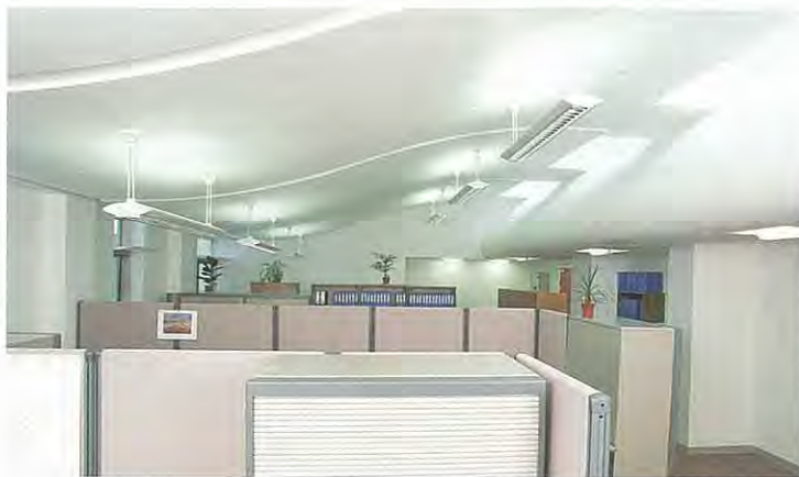
9. Office with high curved ceiling and high level roof vents which dissipate hot air trapped above occupied zone.
