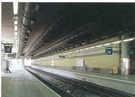
Platforms 5 and 6 central with exhaust ventilation ducting above.
