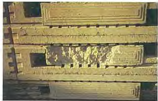
6. The original blocks are weak and friable, with high moisture movement due to absence of coarse aggregate. Wetting and drying can lead to surface breakdown.
