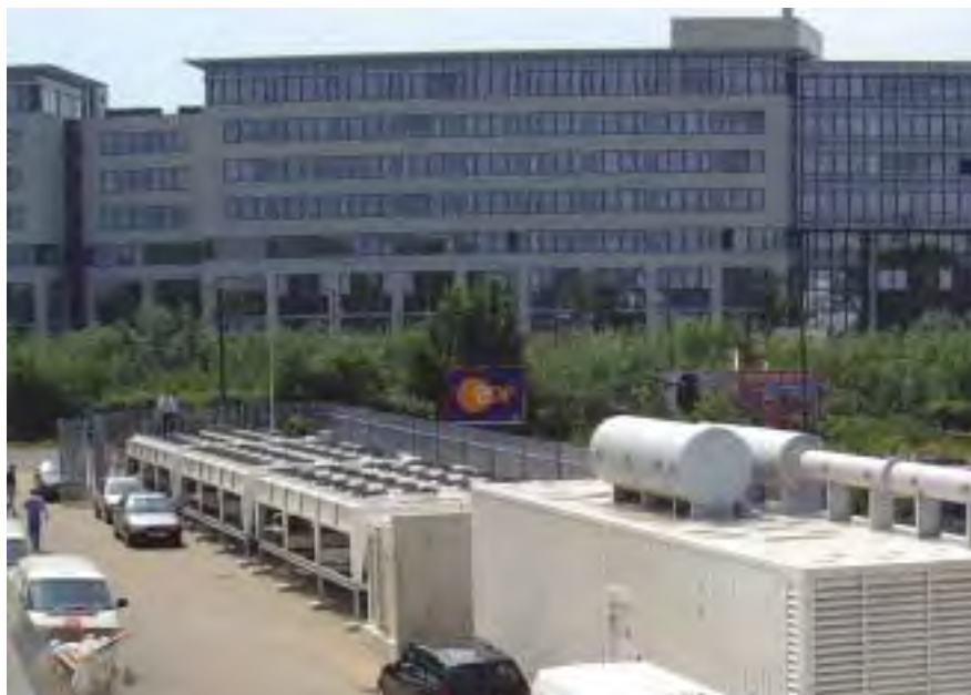
3. External plant at Düsseldorf datacentre.
