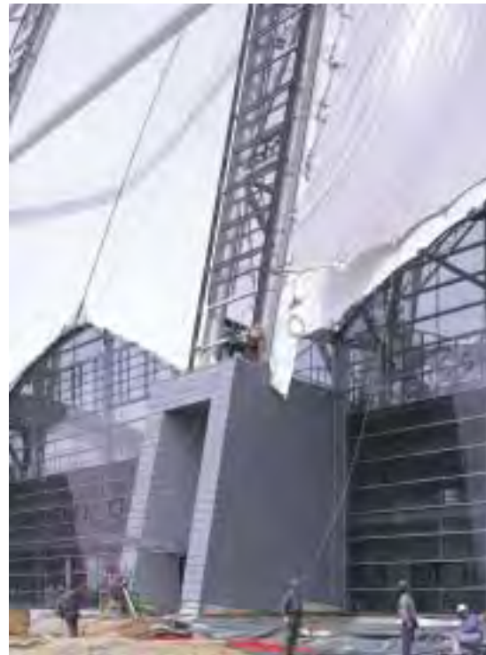
5. One of the building's two main parts: the steel arch-supported, fabric-covered bays. The arches spring from concrete plinths which also act as covered entrances giving protection against snow avalanches.
