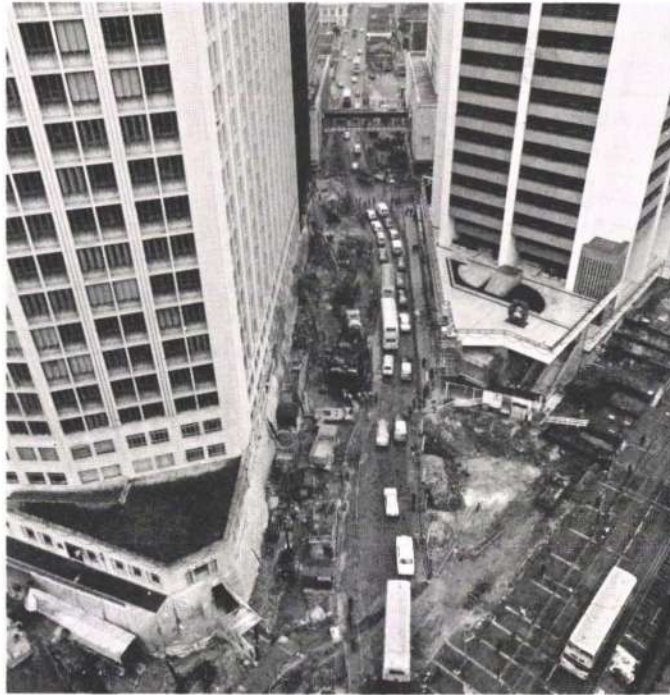
Fig. 21 Construction of the diaphragm wall adjacent to Swire House (Photo: Richard Davies)
