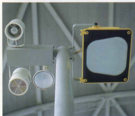
17. Technical tree: carrying fire alarm sounder (top left), public address speaker (bottom extreme left), emergency light (bottom left), light for general illumination (right).
