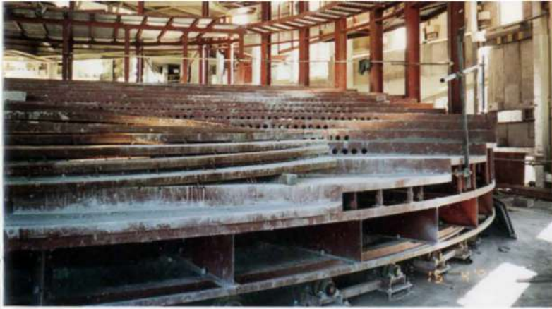
10. The auditorium under construction: the rail supporting one of the rotatable units is visible in the foreground.
