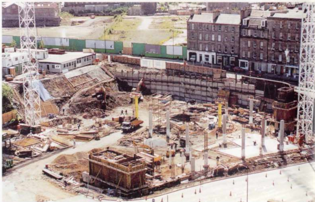
3. The site in May 1993, facing south-east, showing the temporary retaining wall to Morrison Street.
