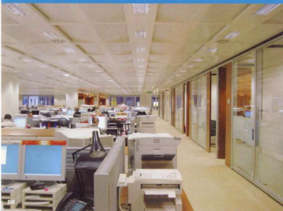
7. Office areas, showing ceilings with multi-service units incorporating lights, swirl diffusers, smoke detectors, and sprinkler heads.
