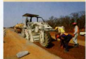
9. Cement stabilization using mechanical self-propelled reclaimer with water bower connected for moisture conditioning during mixing.
