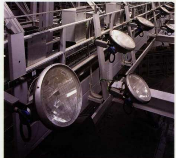
9. Typical floodlighting units.
