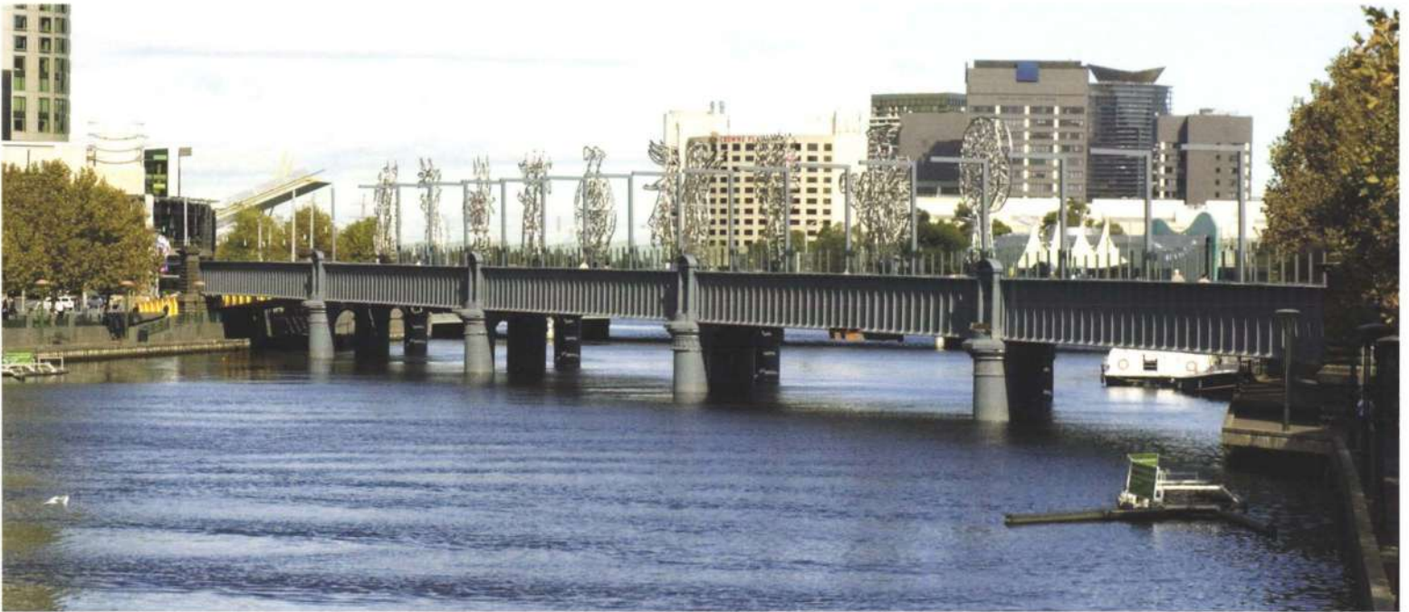
1. Sandridge Bridge with completed Traveller sculptures looking west over the Yarra River.
