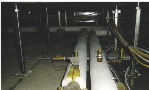
5. Building services run through the raised floor and are easily accessible.
