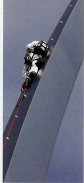
19. Abseiler near the tip of one of the spires. Ropes are attached to engineered clips welded to the back face of each spire to accommodate such access for future testing and inspection.
