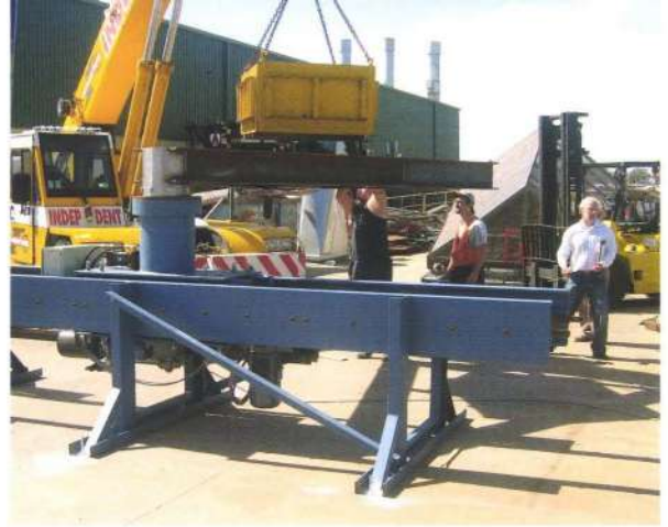
11. Prototype load-testing of Traveller bogies at the Danfab workshop. (Garry Ormsten, project architect, in background).
