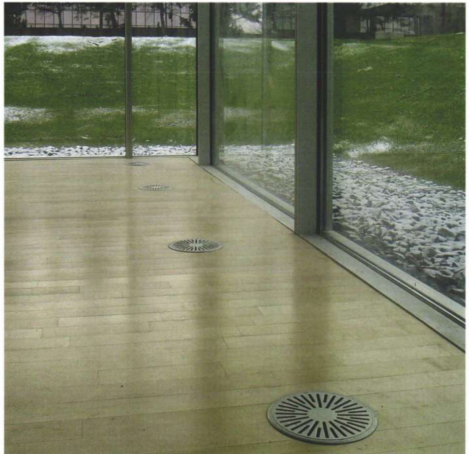
8. Swirl-type floor diffusers are ducted to the FPBs for the conference rooms to mitigate heat gains and losses.
