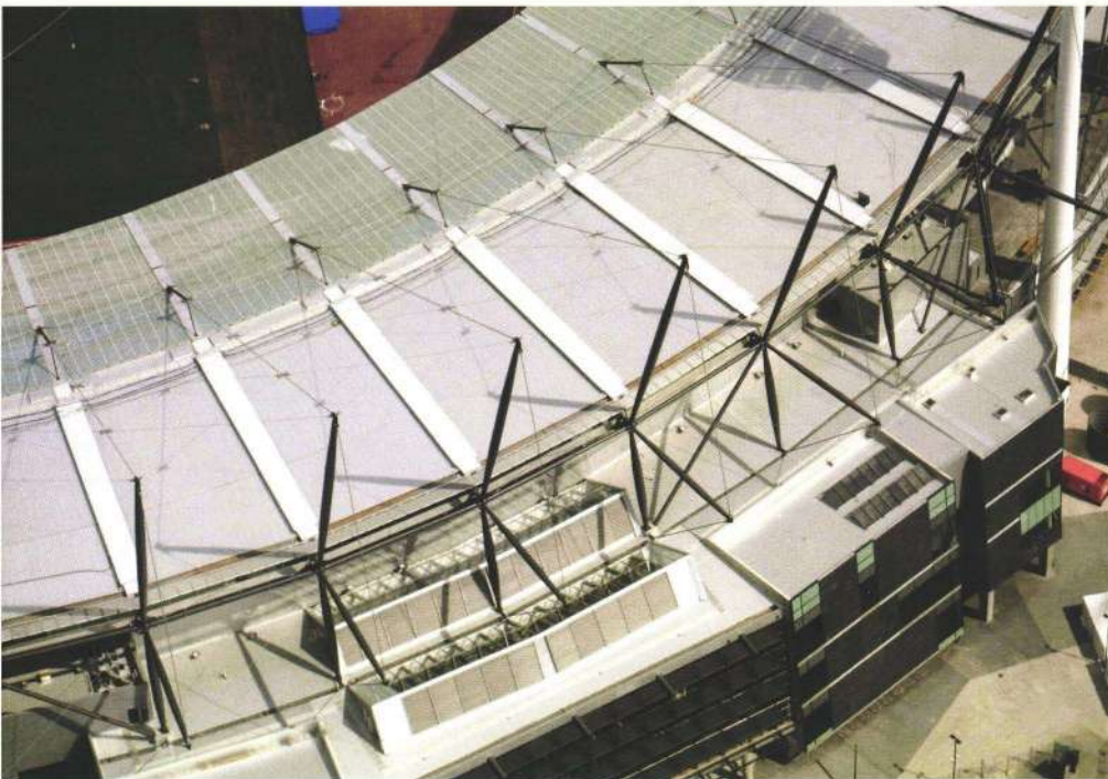
3. The roof is supported from a tension structure with rafters suspended from cable stays running over individual masts and backprops.
