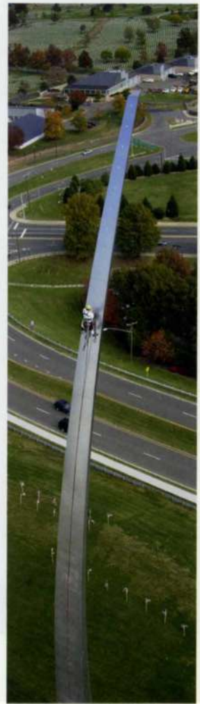
20. A cherry-picker is used to access the first access clip. The abseiler threads his rope through successive clips to prevent the ropes from sliding sideways as he ascends the curve of the spire.
