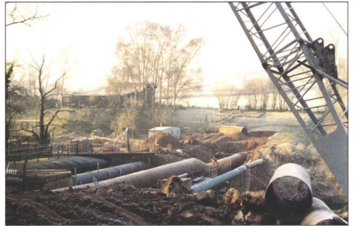
10. Rea River Crossing: The three old pipes are under the canopy on the left of the picture, with work proceeding on installation of the new 60in. main, December 1987.
