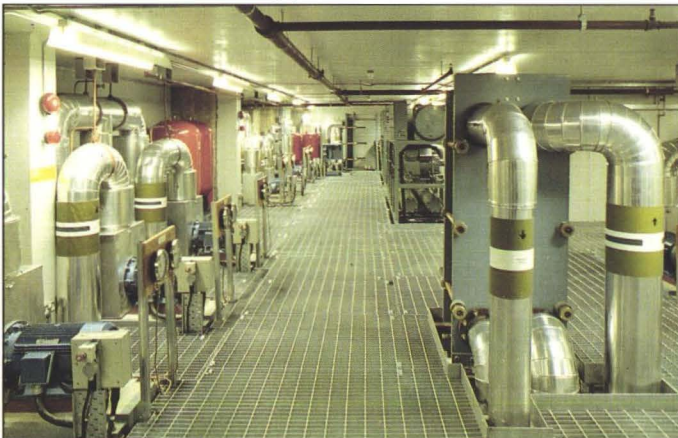
20. Chiller plantroom facing east
