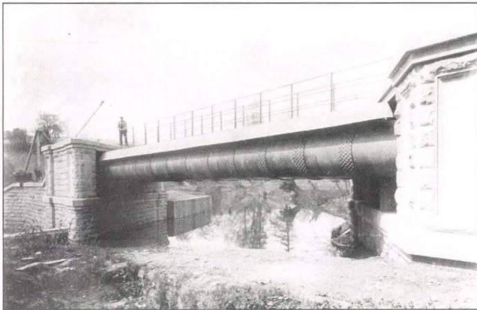
9. Rea River Crossing: Towards the completion of construction in 1902. Three 42in. pipes were installed at this stage.
