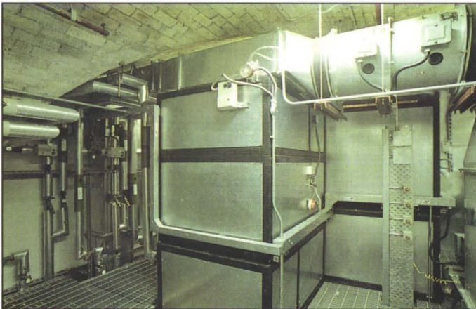
18. One of the 15 air-handling plantrooms
