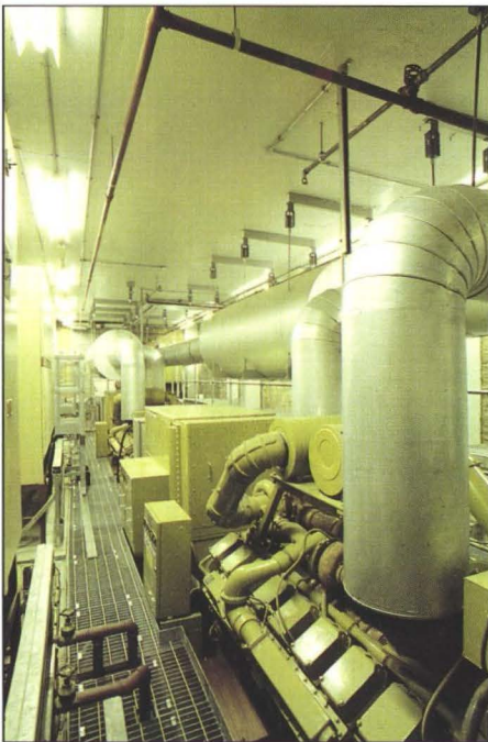
16. Diesel generator room
