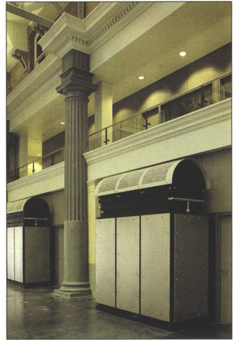
15. Free-standing AHU on ground floor
