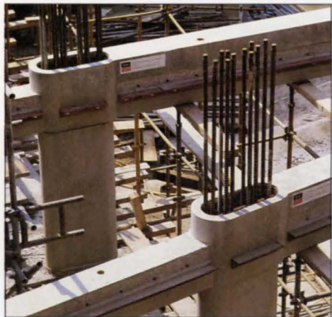
7. Reduced depth beam/column connection showing stepped beam on left, and steel angle floor supports in foreground.
