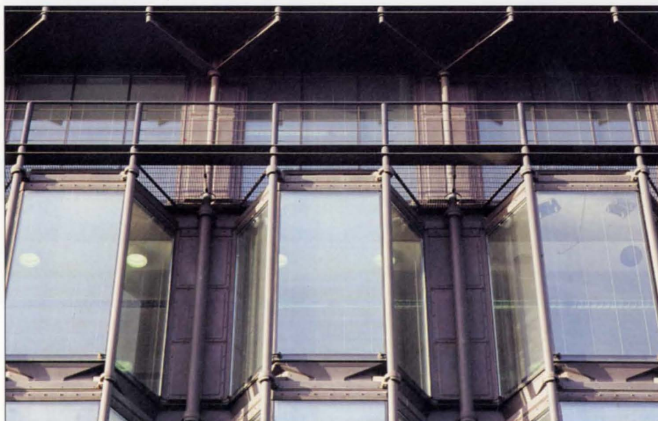
18. Top level of façade. Right 19. Main column on façade with smoke extract door behind.
