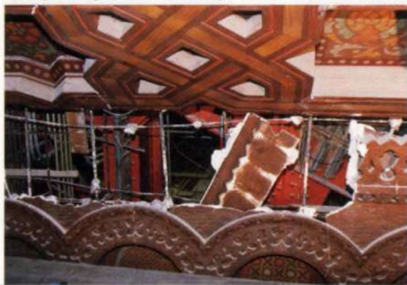
A. Ceiling damage from the Northridge earthquake
