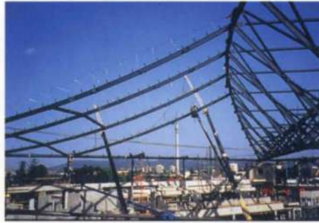
H. 410mm UB catenaries draped from truss to perimeter. 200mm UC arch members follow behind to brace perimeter.
