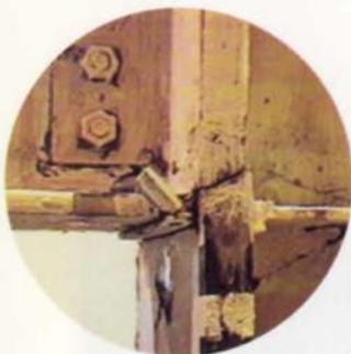
5. 'Pre-Northridge' moment connection: Fracture through column flange.
