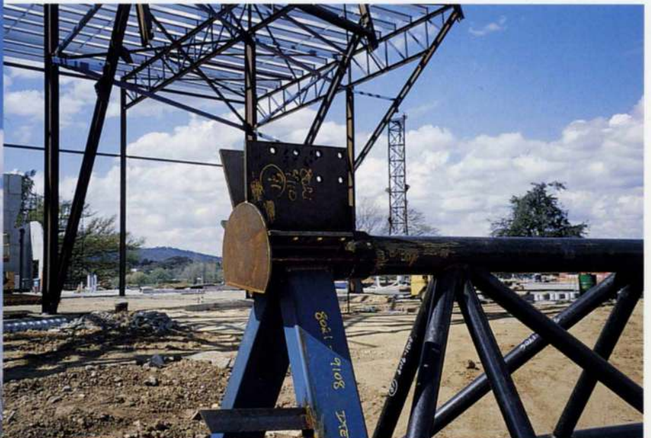
7 above: Foreground: Temporary Gallery structure (in unpainted steelwork, for cost saving) awaiting erection; in the background is the first Main Hall tower.
