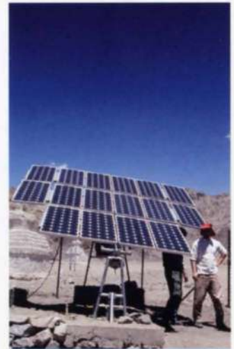
7. Solar panels power water pump.
