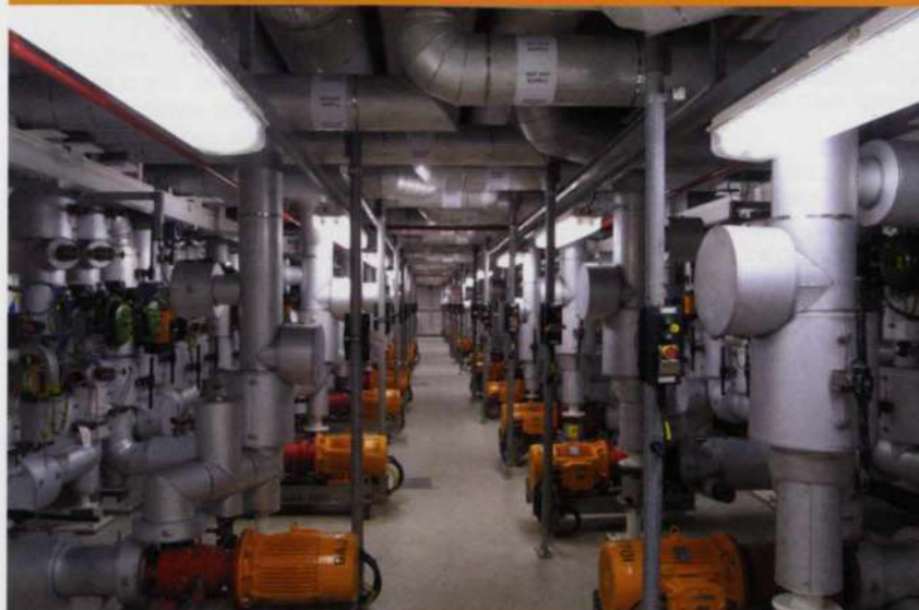
20. Jacket pump room in the production building.
