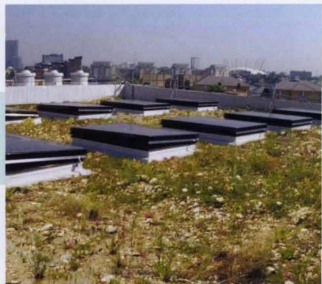
11. Laban's green roof: a protected and undisturbed habitat for the endangered Black Redstart.
