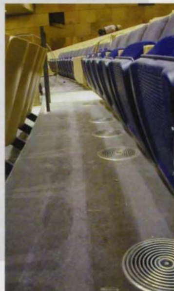
13. Jackson Hall floor diffusers.
