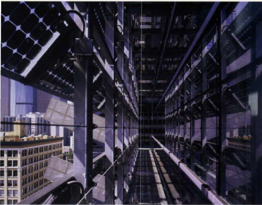
6. View of maintenance walkway on the south façade between glazing and photovoltaic panels.
