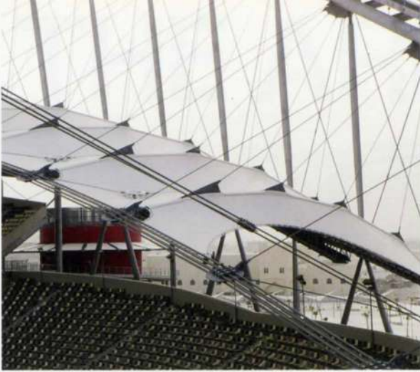
12. Main roof catenary and ridge clamps.
