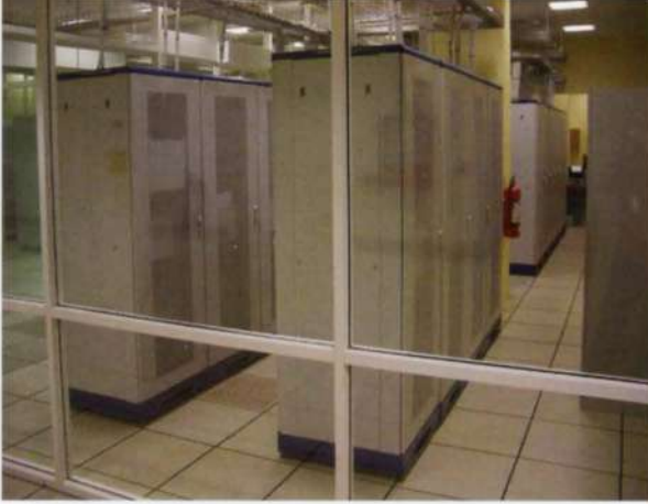
9. The main server room.
