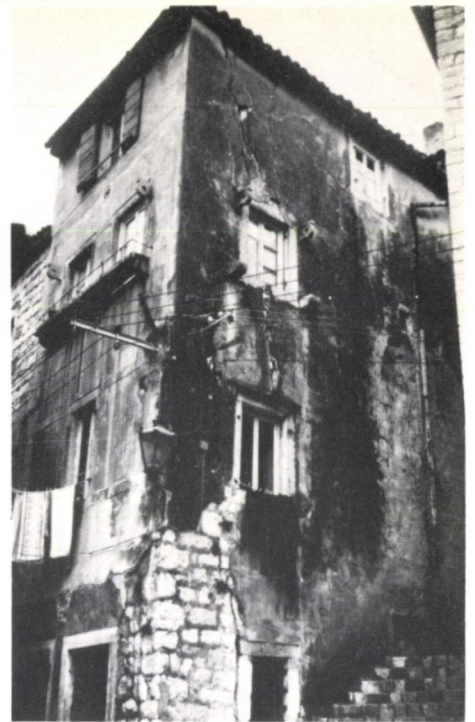
Fig. 8 People have to live somewhere— cracks or no cracks!
