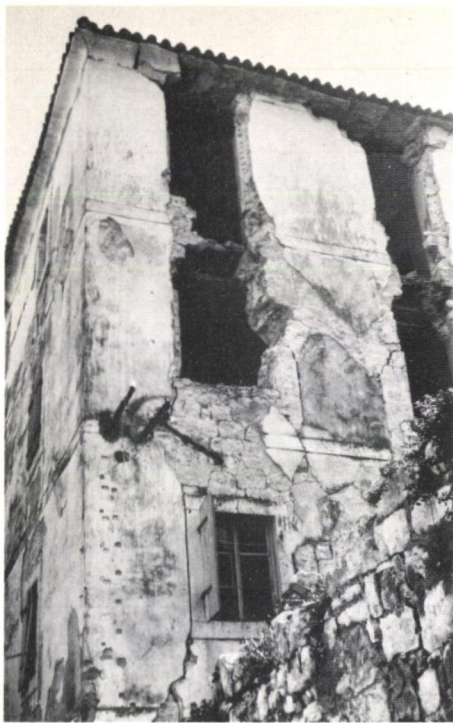
Fig. 3 House in Budva with characteristic pattern of damage
