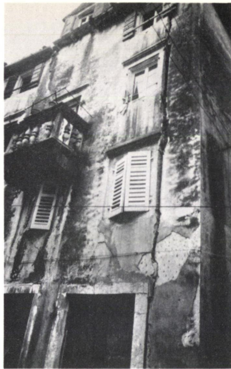
Fig. 4 Kotor: crack following straight joint between stone window surround and corner masonry
