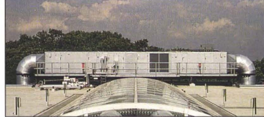
12. View across the roof of one air-handling unit, supported on a gantry above the roof surface.
