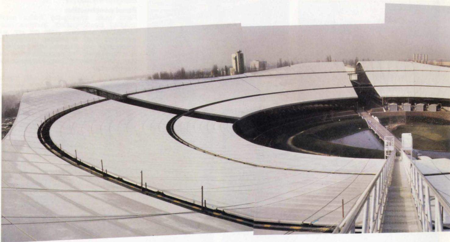
10. Roof nearing completion (panels at cleaning cradle tracks yet to be installed).
