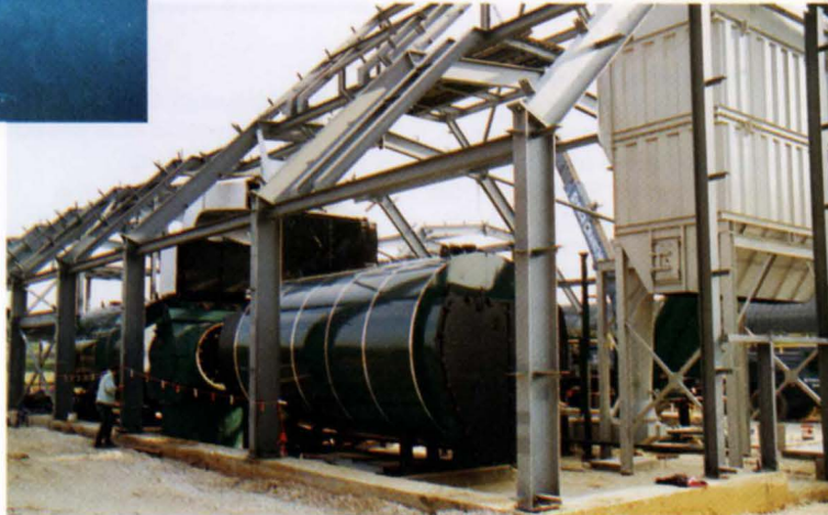
5. Installation of (left to right) flue gas diverter, waste heat boiler, and fabric filter (baghouse).
