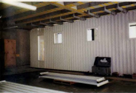
12. Blast protection to computer room.
