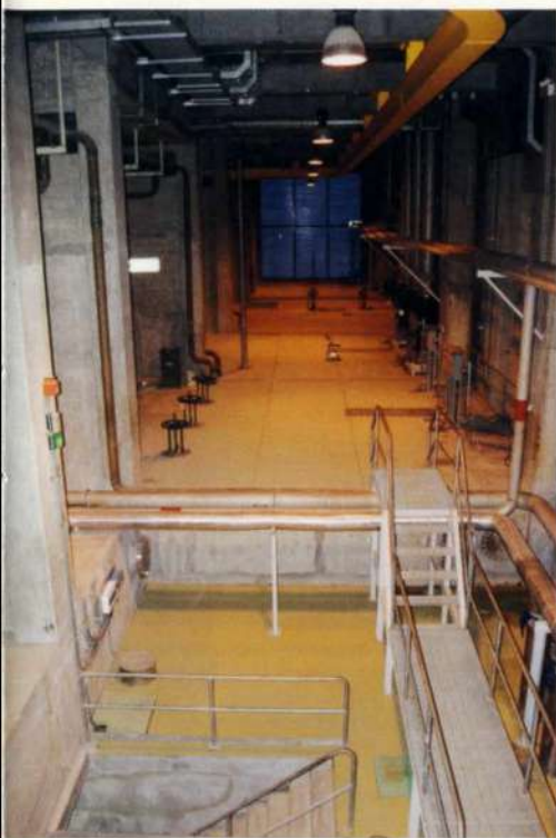
19. Central gallery of treatment plant.
