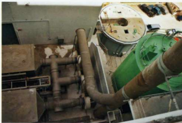
15. Chemical scrubber for odour control.
