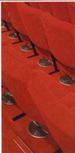
11. Air is supplied to the auditorium via floor diffusers.
