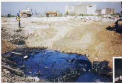
4. 'Hot spot' of contaminated material (tar) encountered during excavation.
