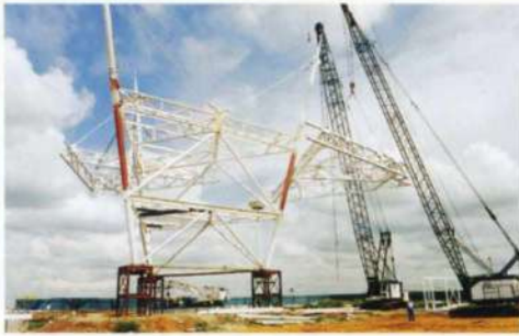
5. Large sub-assembly of node roof being lifted into place in the temporary construction yard.
