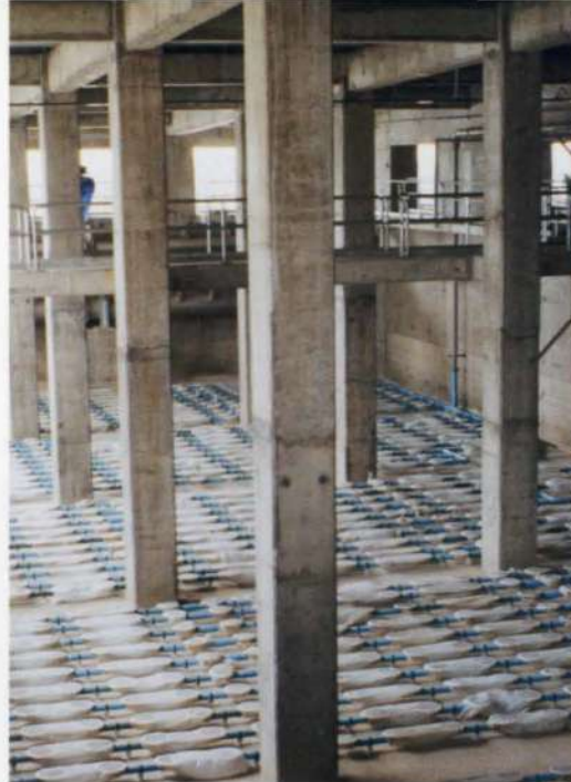
13. Treatment basin, showing bubble aerators.
