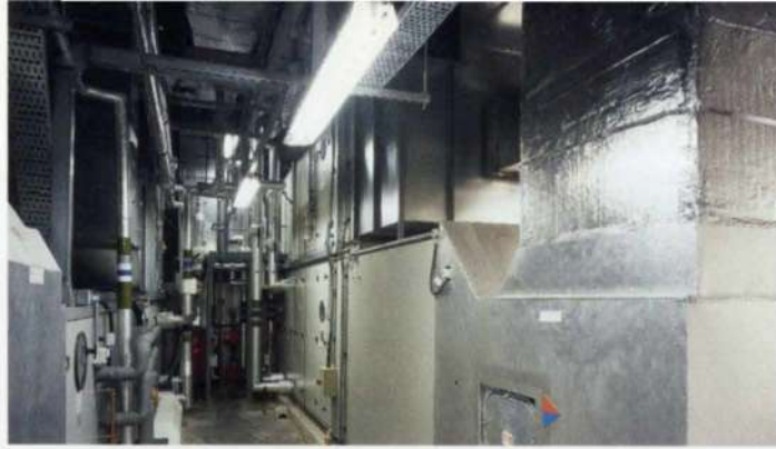
13. Air handling plant at level 1.
