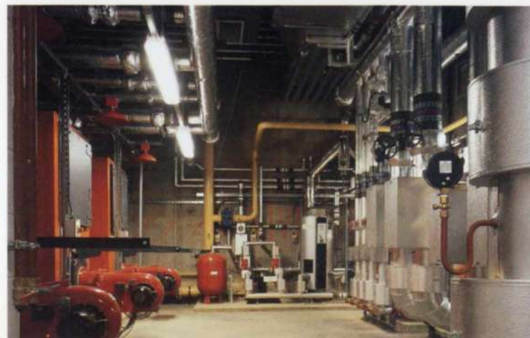
15. Central boiler room.
