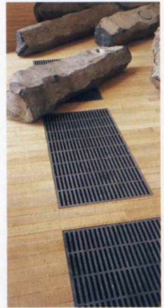
12 below. Air supply to the galleries is via cast iron grilles.
