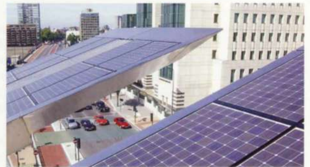
6. PV cells on upper surface of cantilevers.
