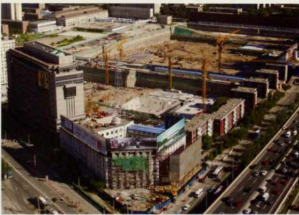
9. Site progress, August 2005: TVCC is in the foreground, with piling completed and excavation to the base of the rafts. Piling is complete at CCTV (behind) with excavation under way to the base of the rafts (up to 30m below ground level).
