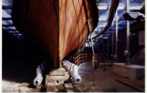
3. Low level dehumidified air supply and high level extract ductwork at the bow.
