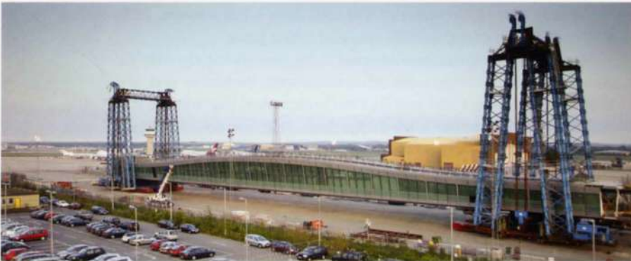
9. The 164m-long deck section with the lifting towers, on the transporters at the prefabrication yard.
