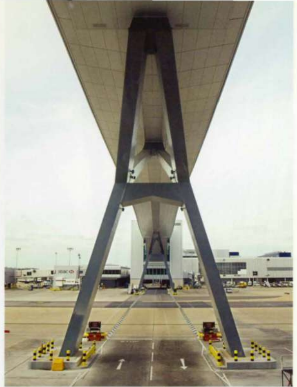
11. In their final position, the scale of the supporting columns is clearly apparent.
