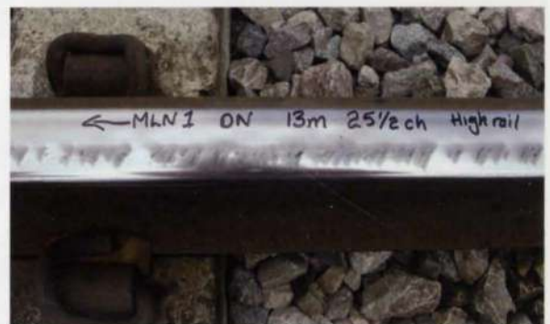
4. Head checking on a 1300m curve.
