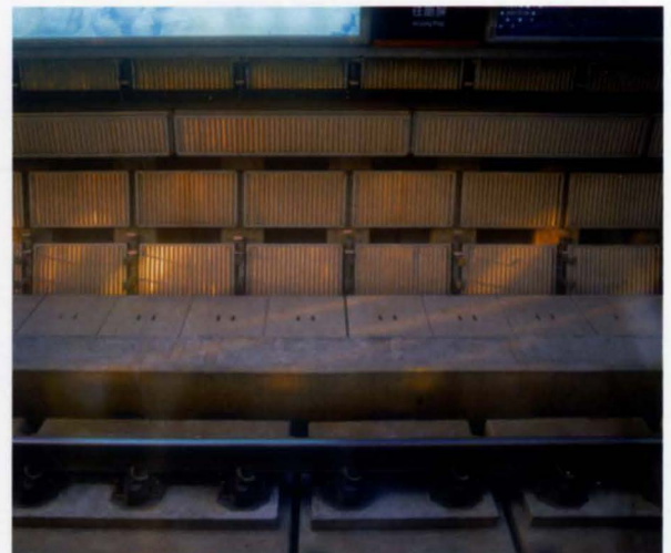
8. Acoustic panels on the parapet.
