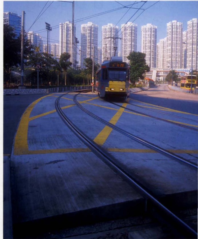
7. Typical road crossing where the trackwork is boxed out within new road slab
