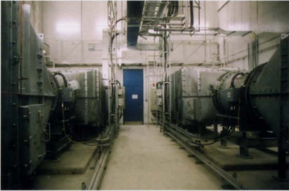
9. Tunnel ventilation plant.
