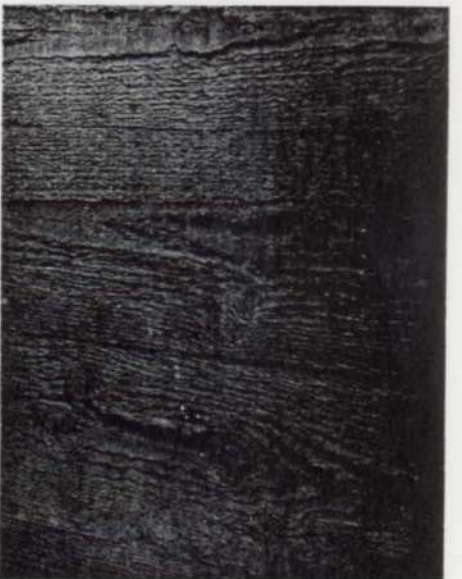
Fig. 3 University of Manchester Economics building. Finish of infill panel. Photo: Ralph Stephenson.
