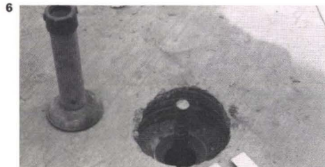
Figs. 3-6 Sequence of rock anchor installations on site for Ministry of PTT Headquarters building (Photos : Robert Pearson)
