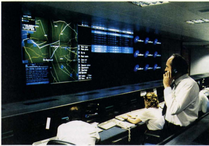
8. Cellnet network management centre. (Photo: Cellnet)
