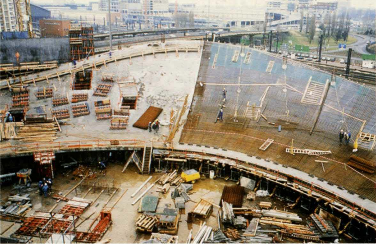
9. Above: Warped gallery floor slab under construction: one half cast, one half decked out with formwork.
