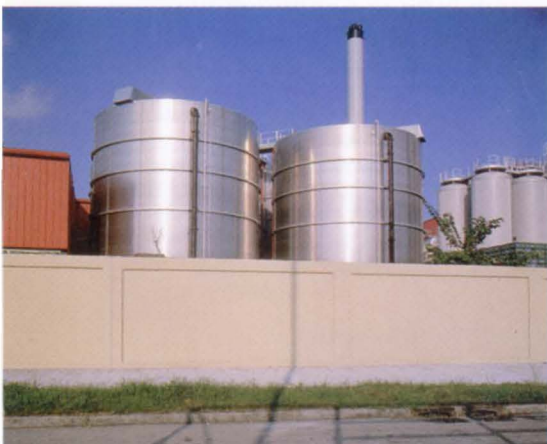
14. Water storage tanks.
