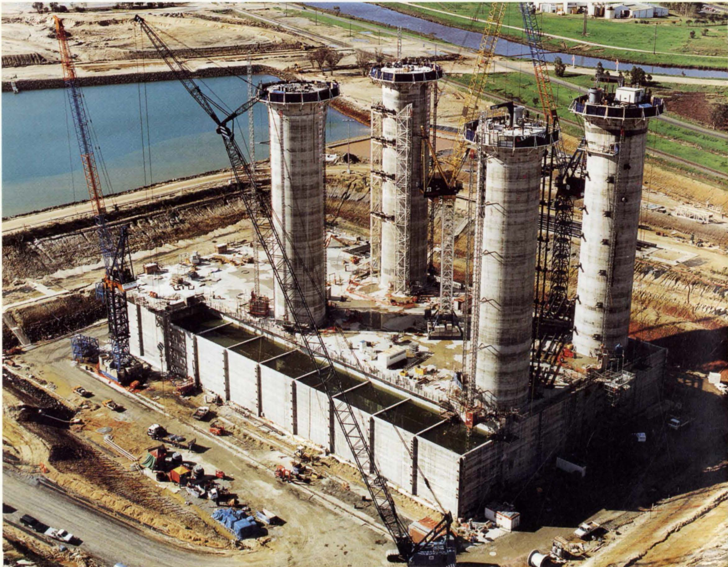
6. The installation in July 1996: eight open cells in foreground, and closed cells behind.
