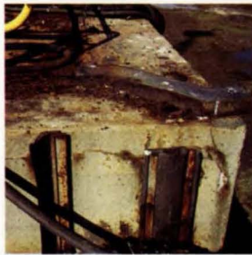
Existing lip and caisson seals on the quoin of the west roundhead.
