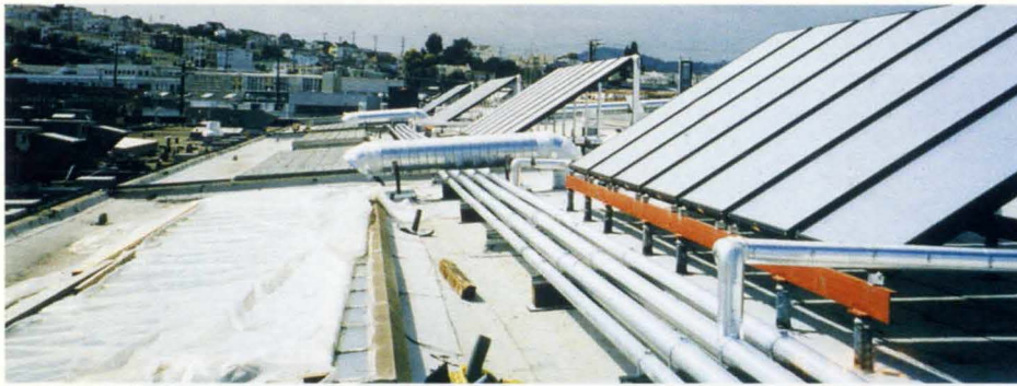
6. Solar panels and skylights on the roof.
