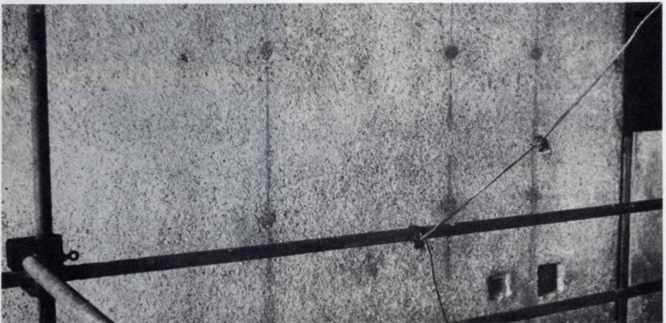
Fig. 4 below Tower Block 1. Staircase wall after bush-hammering; shutter joints and bolt holes still show
