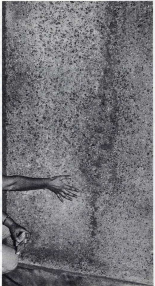
Fig. 5 above Block 11. Typical mark left by shutter joint after bush-hammering
