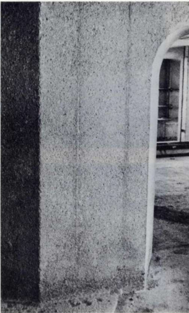
Fig. 3 above Tower Block 1. Lobby walls after bush-hammering; shuttering joints still show.
