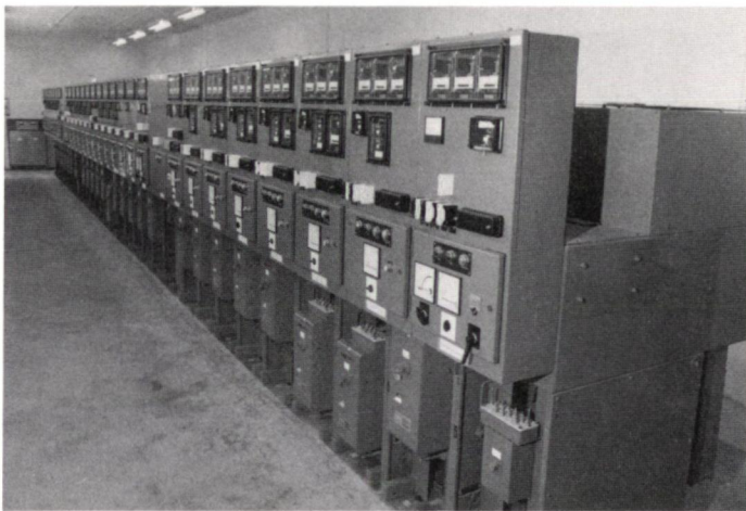
Fig. 40 31 panel 11kV main switchboard
