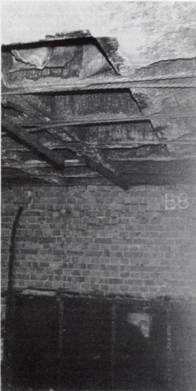
Fig. 6 Damaged soffit waffle slab
