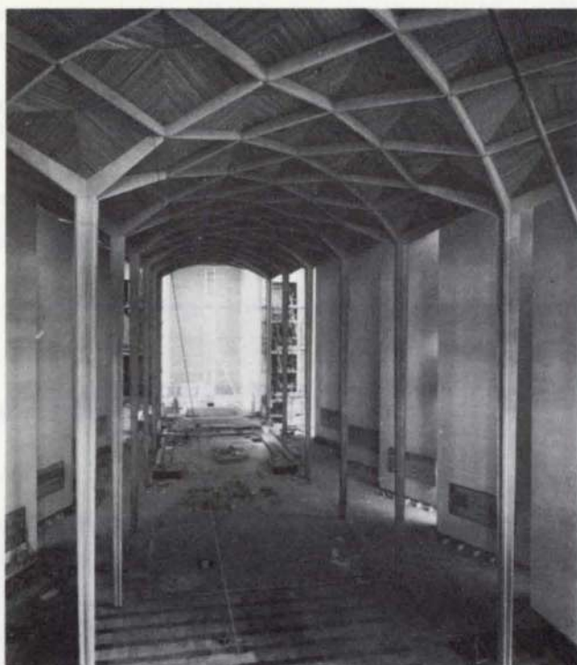
Fig. 1 above Interior view of Coventry Cathedral nearing completion showing the columns and ceiling. The columns were precast in three sections. (Photo: John Laing & Son Ltd.)
