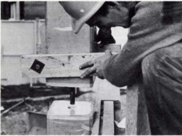
Fig. 8 Forming the joint between precast columns at Somerville College, Oxford University, Phase III. (Photo: Oliver Spence.)
