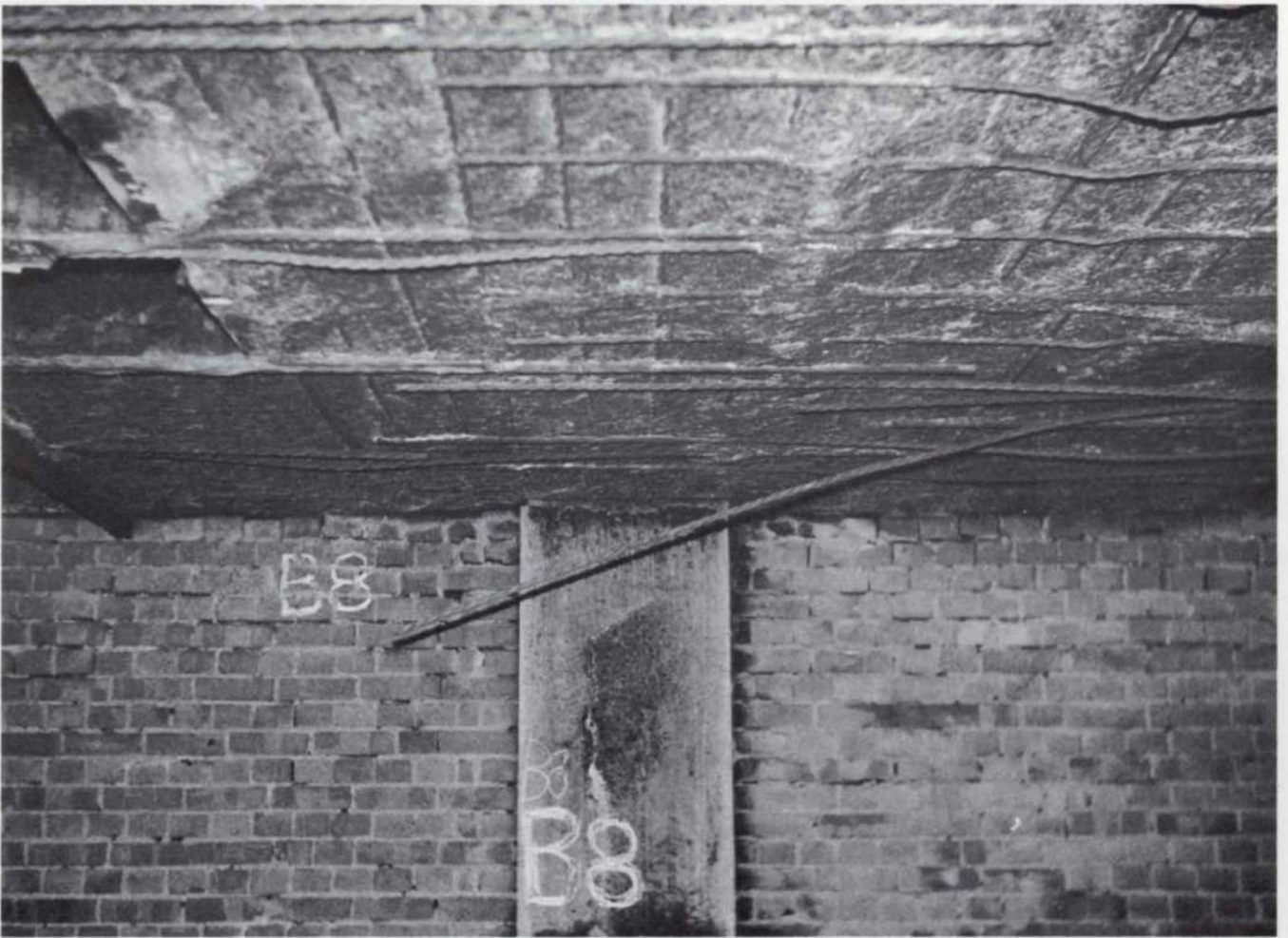
Fig. 4 Damaged soffit solid slab
