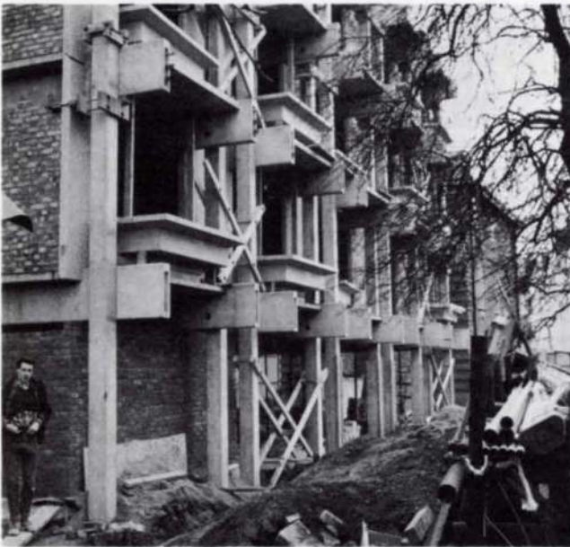
Fig. 9 View of the frame of the Phase III building at Somerville College, Oxford University. (Photo: Oliver Spence)
