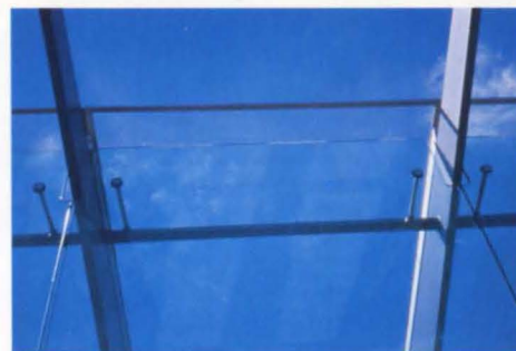
5: Wall installation on footbridge before installation of roof glass, illustrating restraint bearings to top of glass fixed on hollow section restraint.
