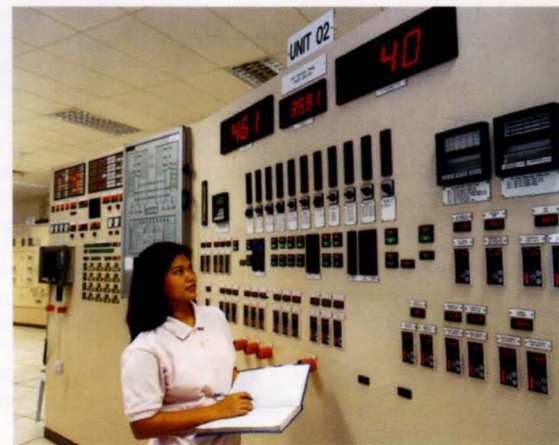
12. Central control room.
